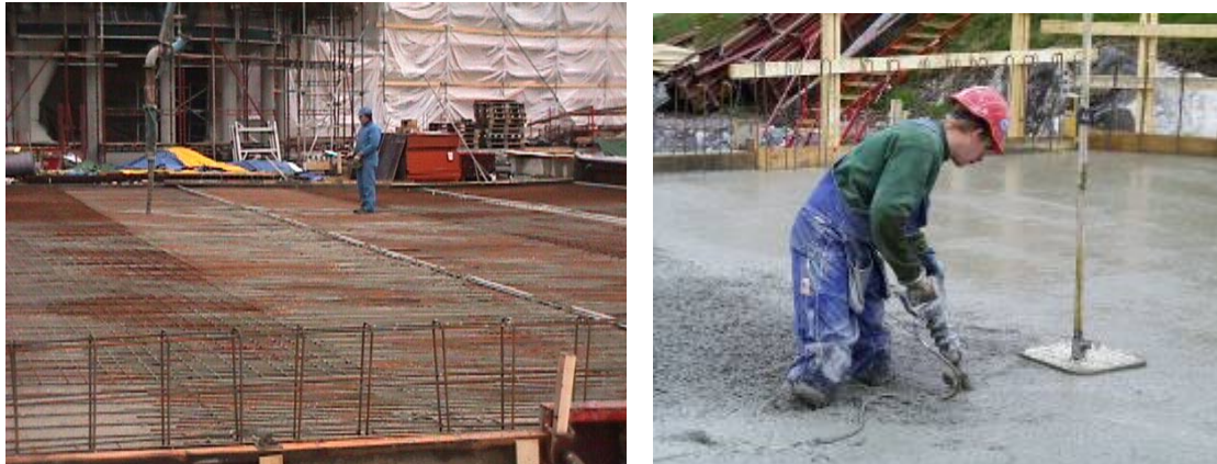
Figure 4 Which technology would you prefer for casting a slab? Choose SCC (left) or a situation you might land in with traditional concrete (right).
